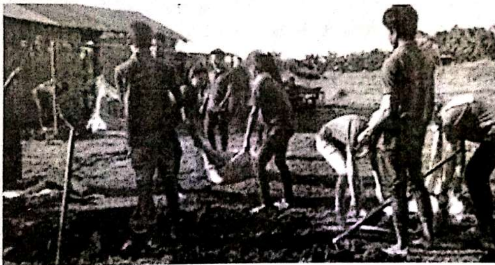
A view of NSS volunteers repairing the bamboo bridge and school of the adopted village.
