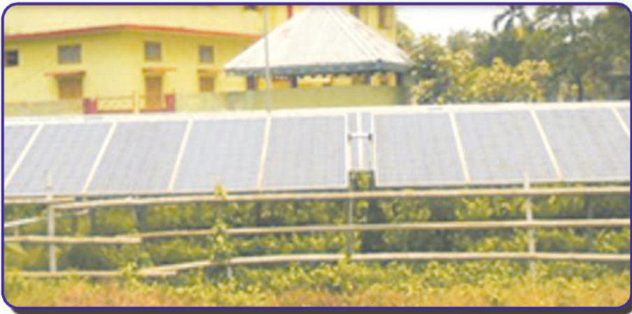
50 KWp Solar Power Generator
